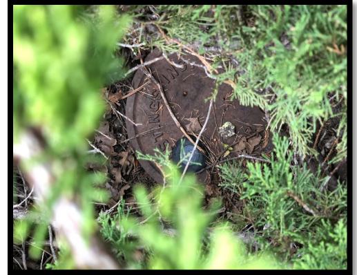
An example of a meter pit that is not well-maintained Photo courtesy of Pinery Water Staff.
