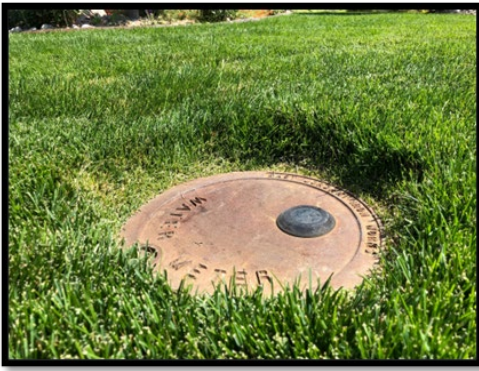
An example of a well-maintained meter pit. Photo courtesy of Pinery Water Staff.
