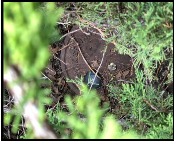
An example of a meter pit that is not well-maintained .
