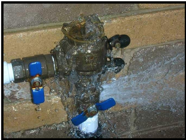
Picture from: https://www.colorado.gov/pacific/evergreenmetro/news/winterizing-your-sprinkler-system
