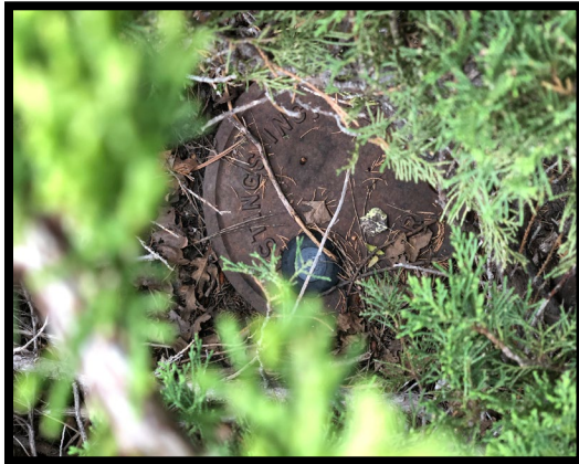
An example of a meter pit that is not well-maintained Photo courtesy of David Chatagnier
