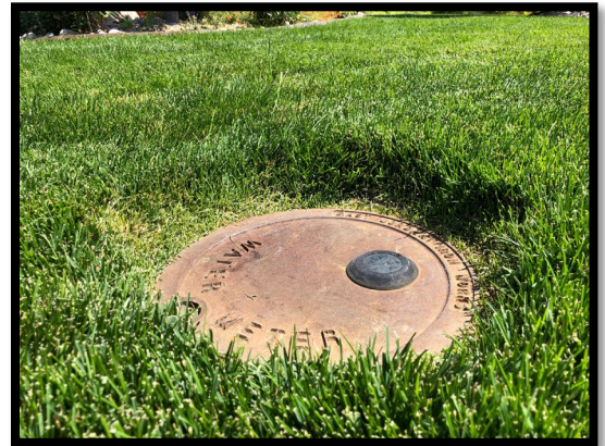
An example of a well-maintained meter pit. Photo courtesy of David Chatagnier
