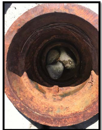
Debris obstructing a valve box prevents a valve from being opened or closed
