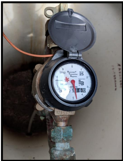
Meter installed in Pinery Water District photo by David Schmitt
